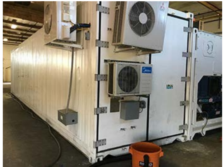
The rear exterior of a Local Roots prototype container farm.
